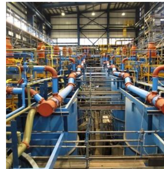
Flotation building piping
